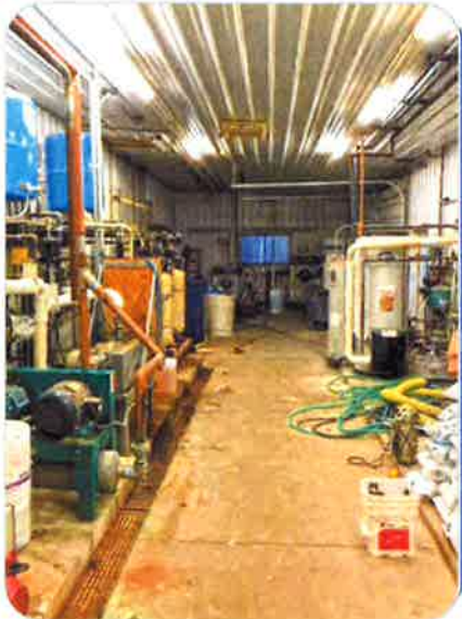
Pump Room Area
