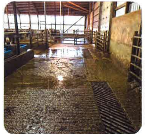
Temporary manure storage system with pump to manure pit
